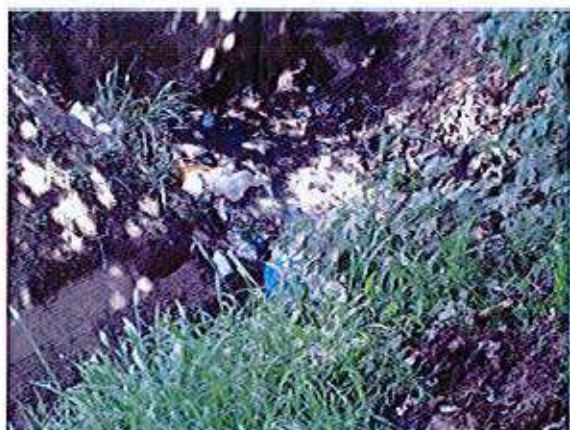
Garbage blocking a water tunnel
